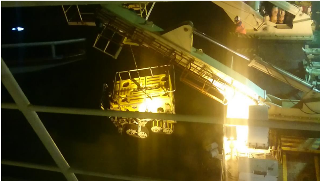
Figure 27 Deployment of the ROV with TSS system during cable repair works near Cornish coast
