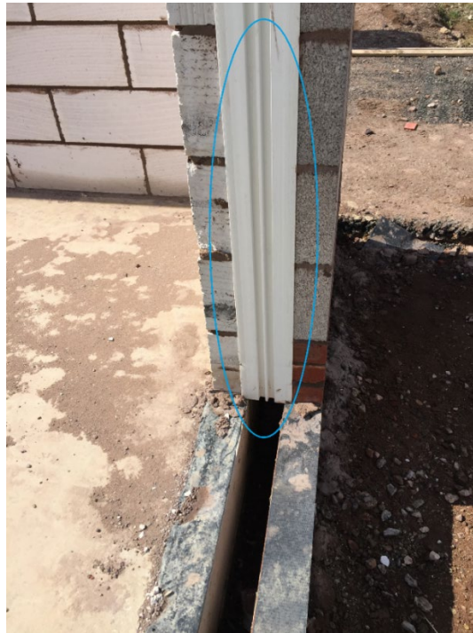
Figure 4-25 Cavity closer installed blocking the identification of defects in the wall's cavity (Source: Taken by this thesis' author)
