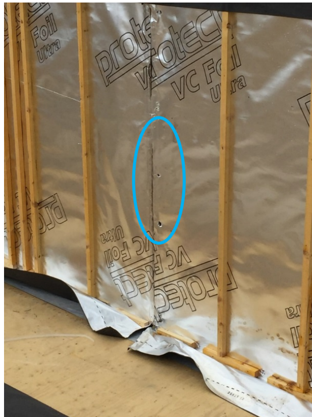
Figure 4-42 Ruptures in vapour control layer in Case study 2 (Source: Taken by this thesis' author)
