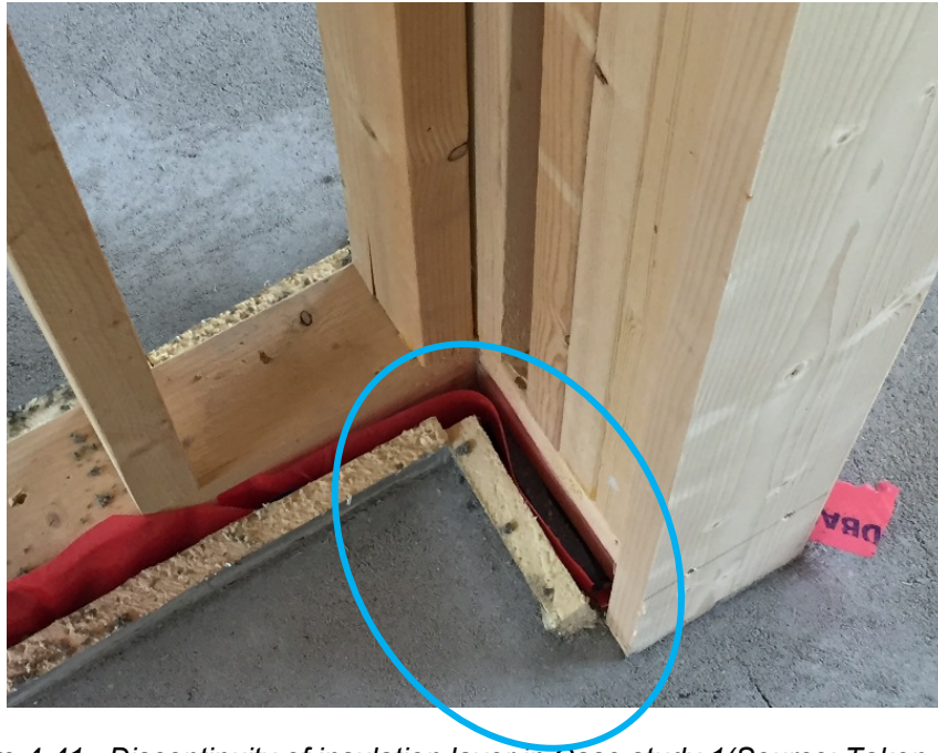
Figure 4-41 Discontinuity of insulation layer in Case study 1 (Source: Taken by this thesis' author)
