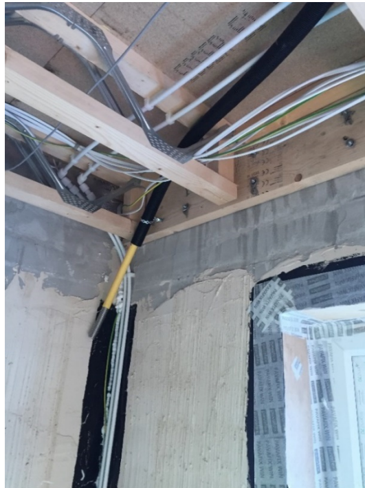
Figure 4-34 Defect potentially affecting air tightness undetected (Source: Taken by this thesis' author)
