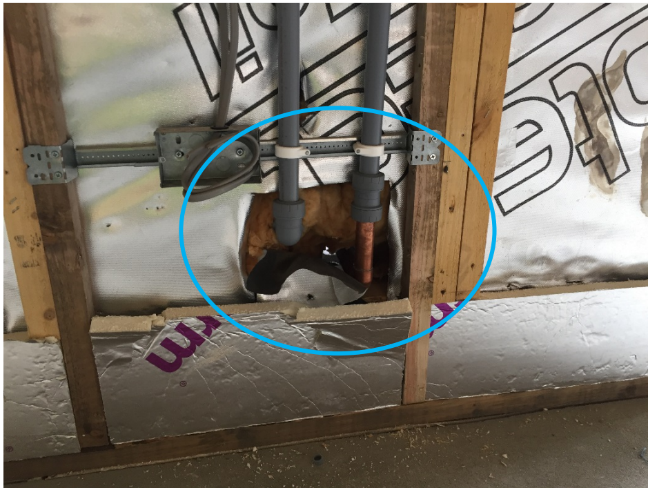
Figure 4-40 Discontinuity of insulation layer and ruptures of vapour control membrane in Case study 1 (Source: Taken by this thesis' author)
