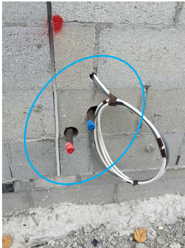
Figure 4-44 Missing insulation around pipes in Case study 5 (Source: Taken by this thesis' author)
