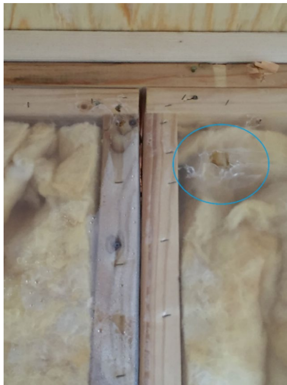
Figure 4-12 Ruptures in vapour control membrane identified in Case study 1 (Source: Taken by this thesis' author)
