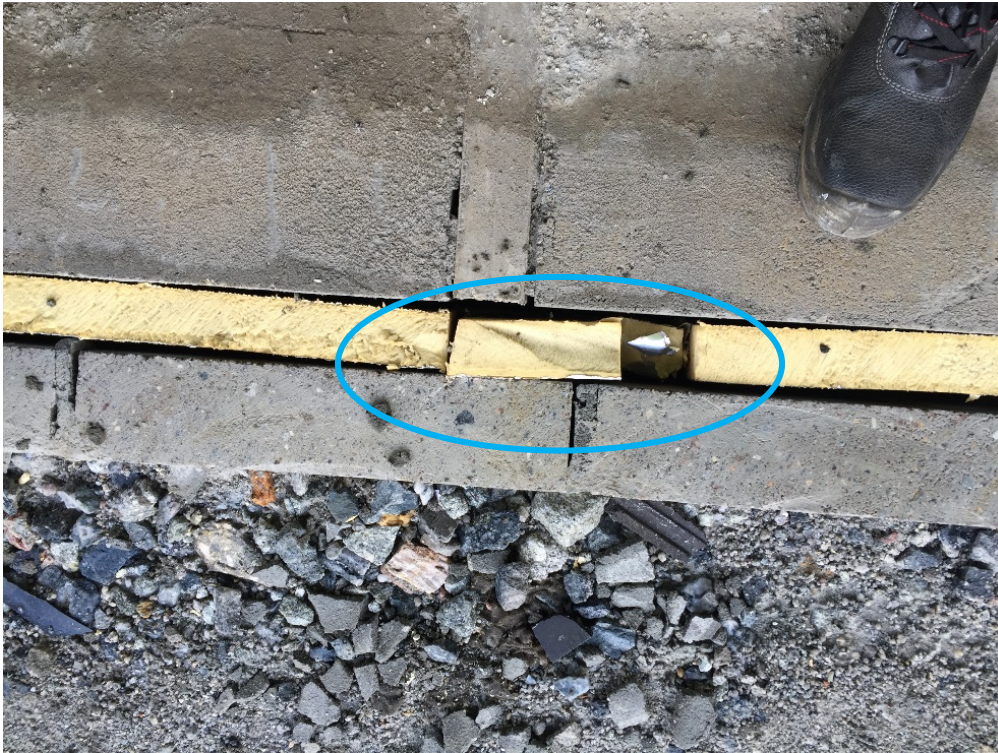
Figure 4-39 Ill-fitted insulation layer presenting air pockets and gaps in Case study 2 (Source: Taken by this thesis' author)
