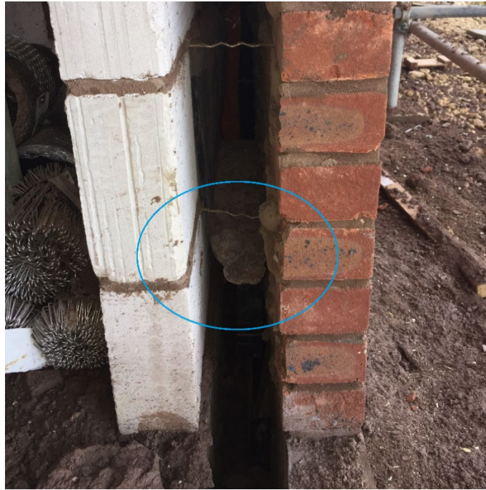
Figure 4-13 Thermal bridging due to debris in cavity tray identified in Case study 5 (Source: Taken by this thesis' author)
