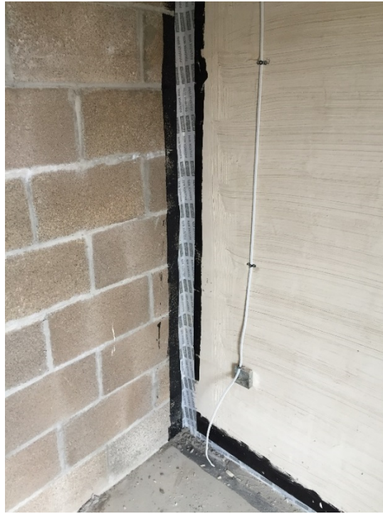
Figure 4-33 Application of air tight tape over primer coat to overcome the risk of cracks of the parge coat in wall corners (Source: Taken by this thesis' author)
