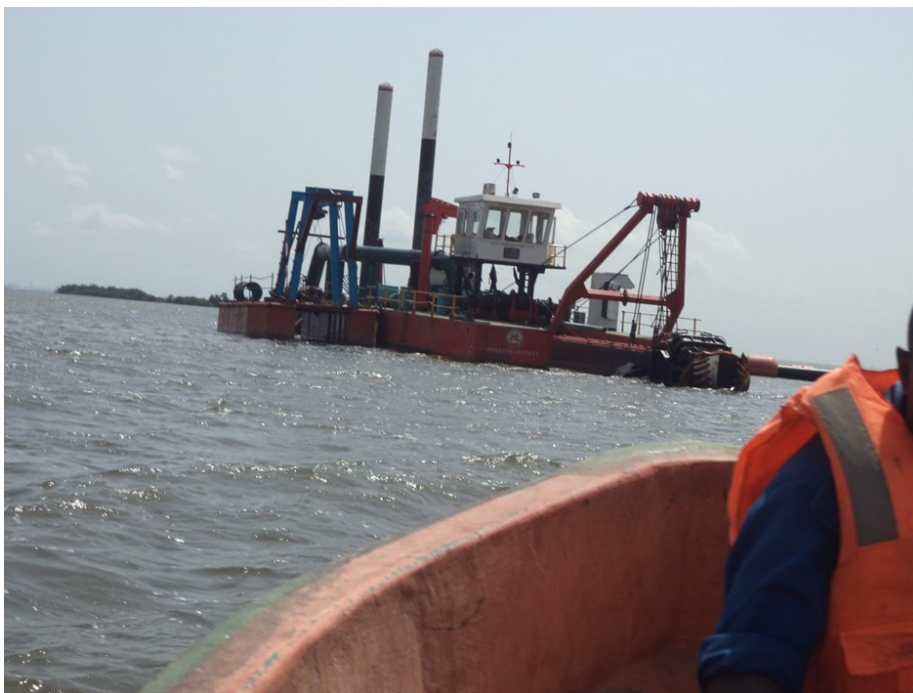
Dredger in one of the area subjected into dredging for the purpose of collecting sand for construction purpose in some sites within the Lagoon ecosystem
