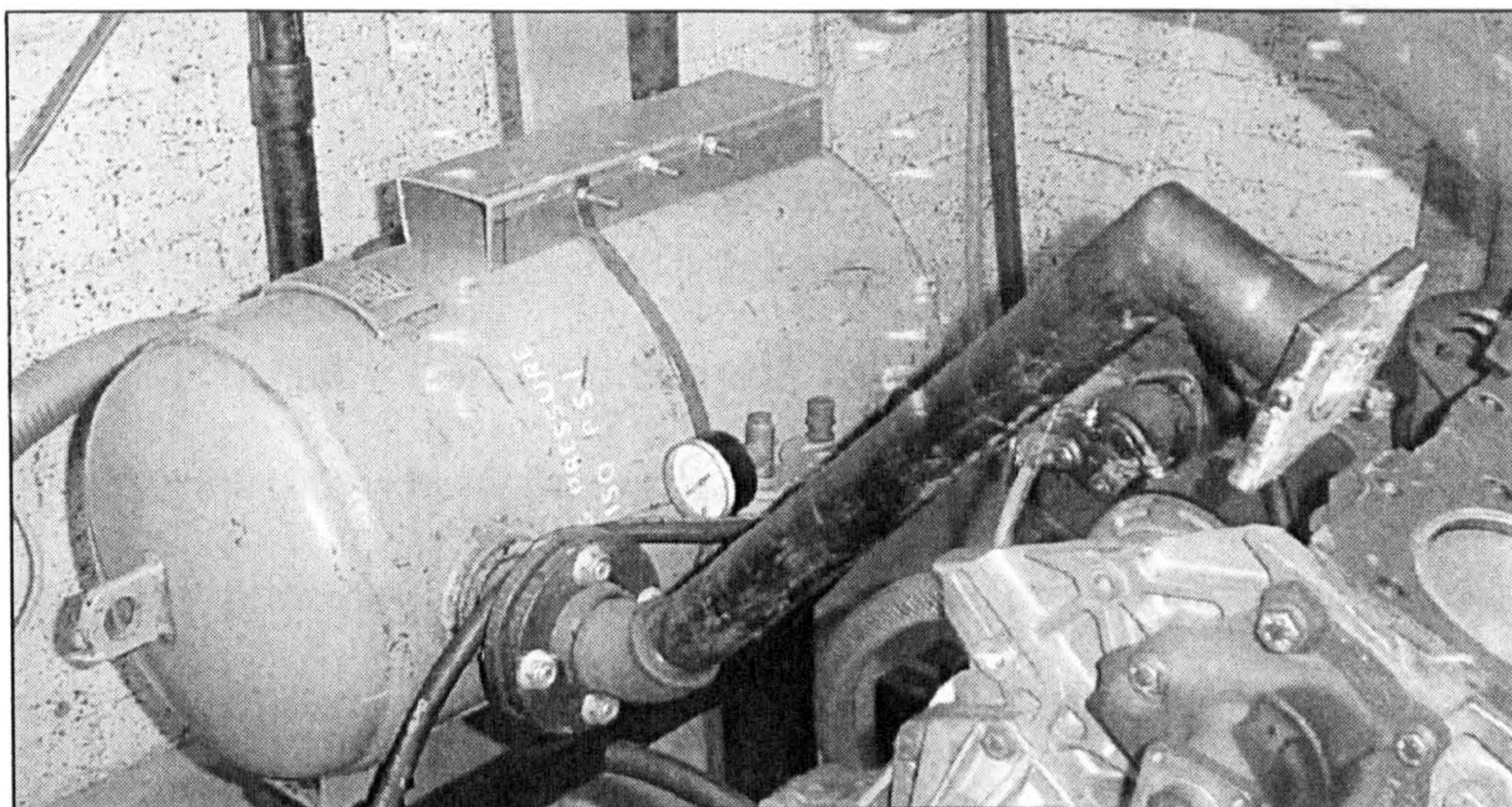
Fig 4.3 Compressor Air Receiver Vessel
