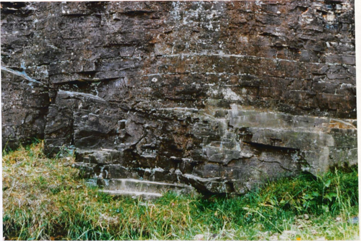
Plate 2.13 Low angle normal fault within the Carboniferous rocks to the north of Plymouth; St. Mellion area [SX 3890 6550]. Height of rock face 1.5m.
