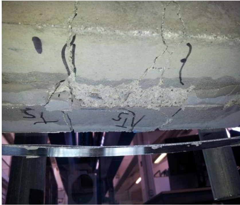
Figure 5.10 CFRP debonding (EBR beam bottom face)
