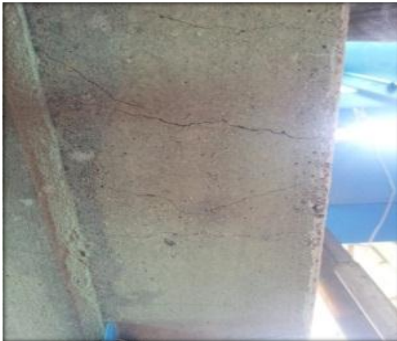
Figure 5.11 Beam cracks (NSM strengthened beam bottom face)
