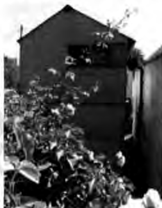
Fig. 2. Building 1, with a thermal probe inserted in the foundation blocks 120 mm below the damp-proof course, supported on a boom stand
