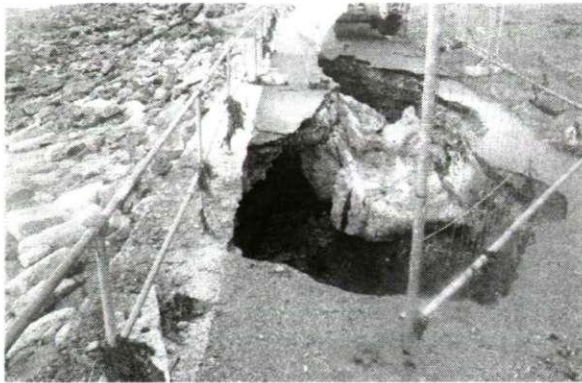
Figure 1.1.3 Newlyn: Damage to promenade due to wave overtopping (Source: Cornwall City Council)
