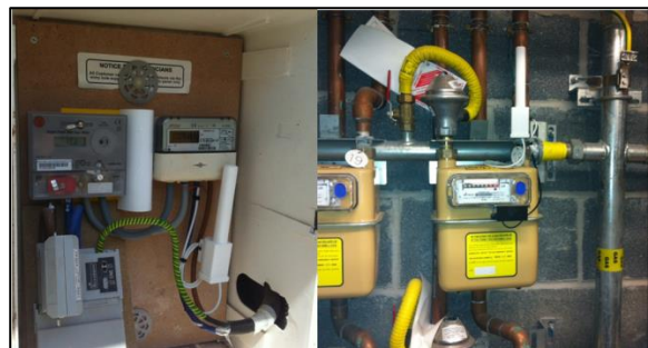
Figure 4 Pulse output sensors connected to the electricity meter (left) and gas meter (right)
