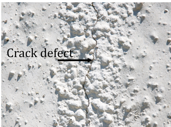
Figure 74. Photograph of crack defect.
