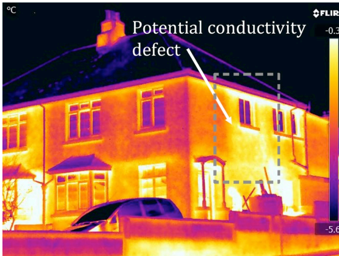
Figure 39. Potential conductivity heat loss through external wall. Dotted box corresponds with figure 40 below.
