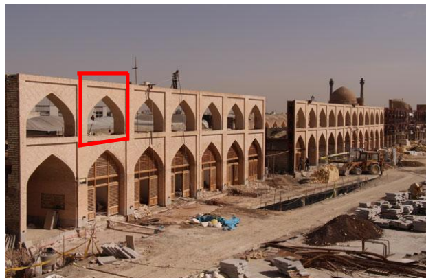
Fig 3.7. Atiq square project (Second phase under progress, 2012) [54] , The highlighted parts in this photograph is showing the Safavid arches in construction of the Atiq square
