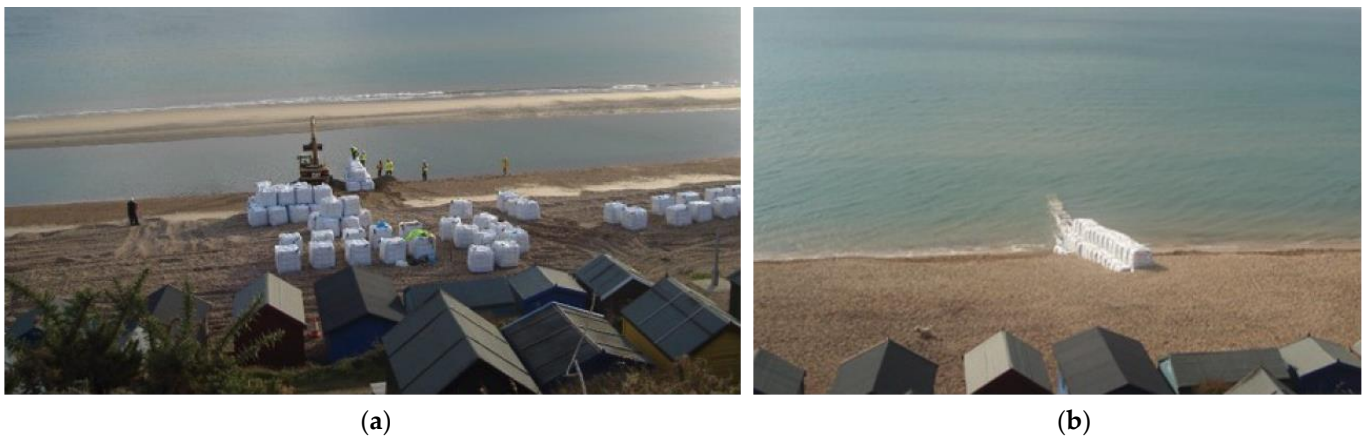
Figure 3. Pictures from the top of Hordle Cliff of (a) groin construction, filling the geobags during low tide on 27 September 2007; (b) view of the temporary structure deployed at Milford-On-Sea.
