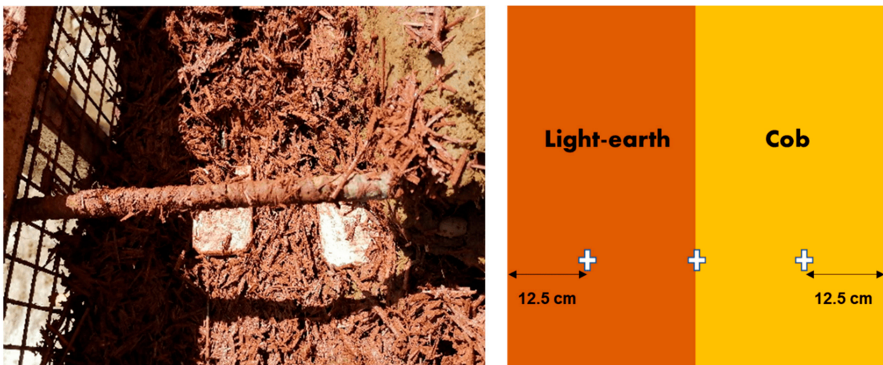
Figure 5. Position of the volumetric water content sensors in the prototype building's walls.
