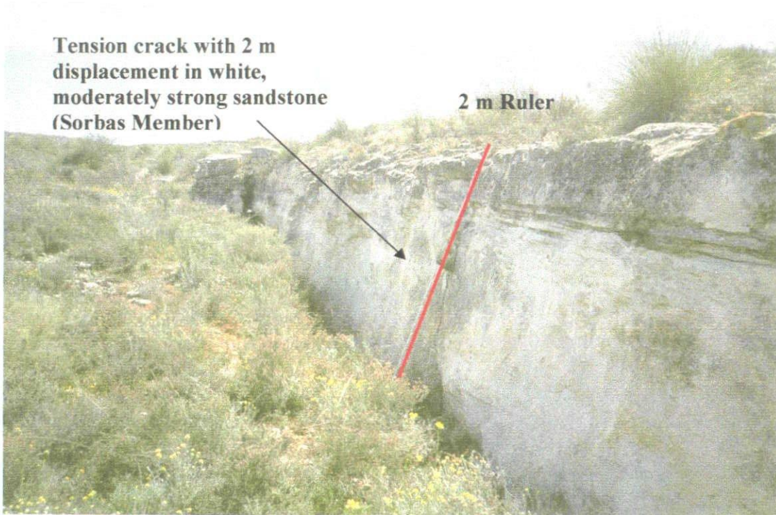
Figure 5.9 – Photograph of the tension crack and backscar associated with the displaced block shown in Figure 5.8 (Grid Reference: 0578041056).
