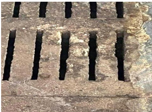
(a) Damage and corrosion of slab
