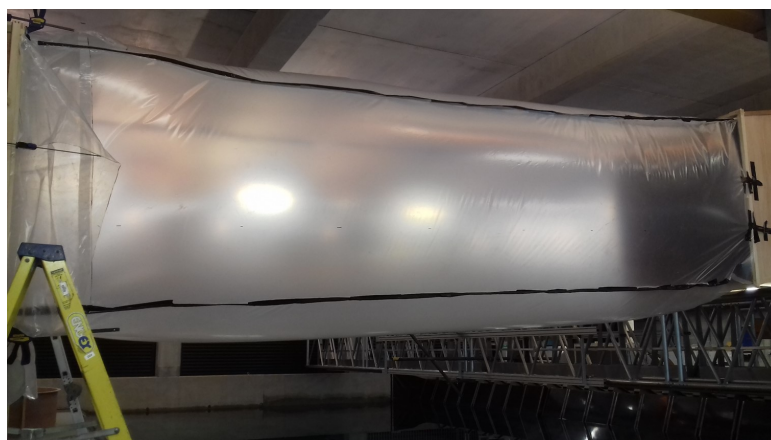
Figure 5.32: Polythene duct guiding air from wooden structure which combines air flow of the two fans to the diffuser
