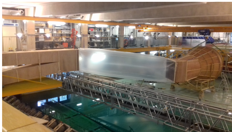
Figure 5.50: Ducting system from fans to outlet
