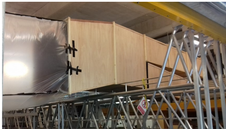
Figure 5.31: Wooden structure to combine the air flow of the two fans
