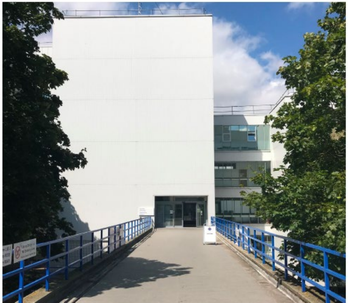
Figure 4.20 Entrance to science buildings; above shows original appearance with austere tiled facades: below shows same entrance with composite panel replacement facade
