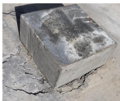
Figure 5. Penetration of column at the top surface of slabs.
