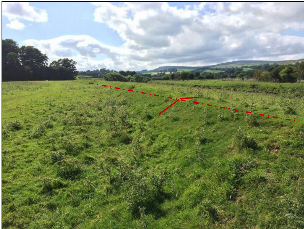
Figure 4-13 Photograph showing a length of embankment alongside reach PR006, as observed during field data collection
