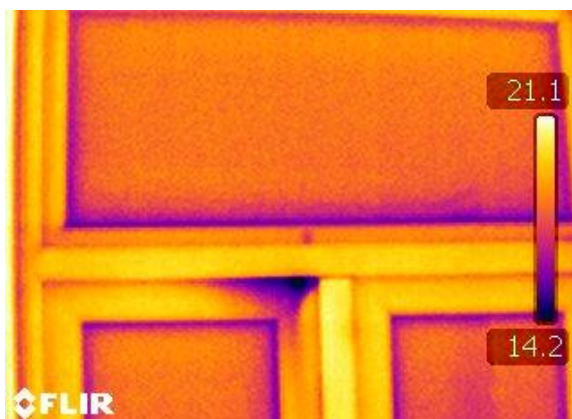
Figure 6.4: Thermal image showing the draught of cold air entering the house where the door has warped at the top.
