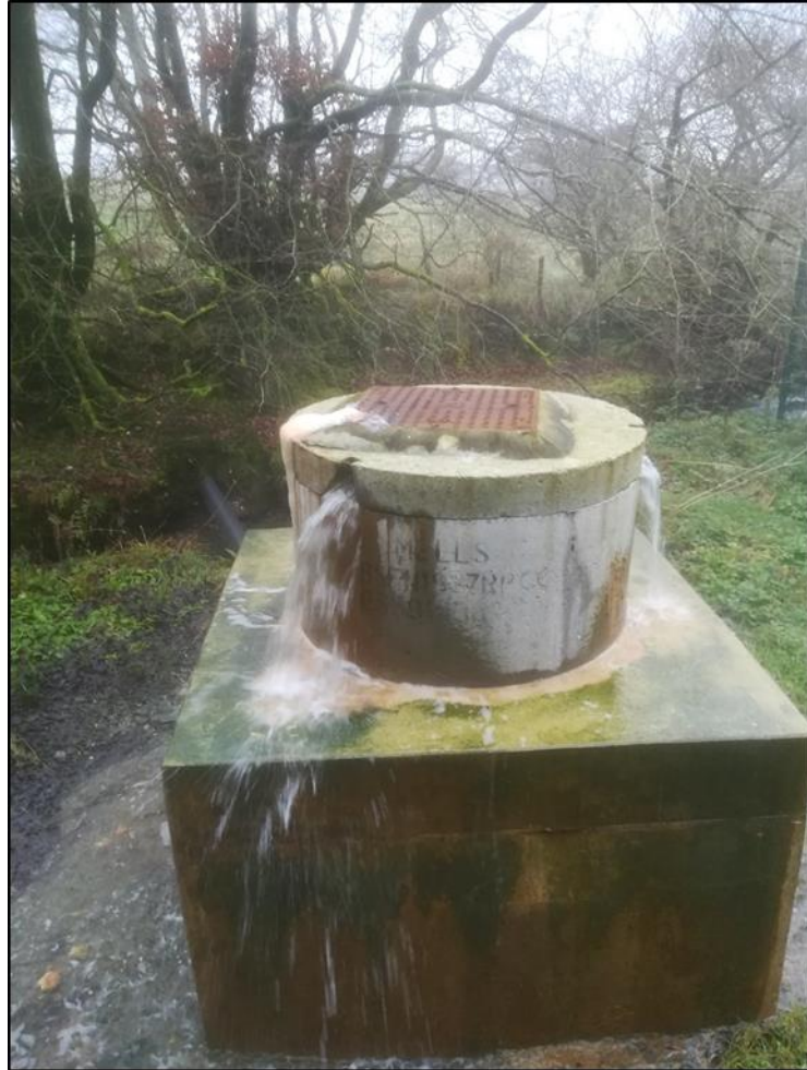
Figure 3.3 Outfall drain overflow at Inny Vale, November 2019
