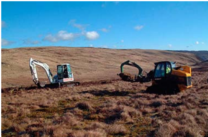
Drain blocking at Lake Vyrnwy using heather bale and peat dams © LIFE Active Blanket Bogs in Wales
