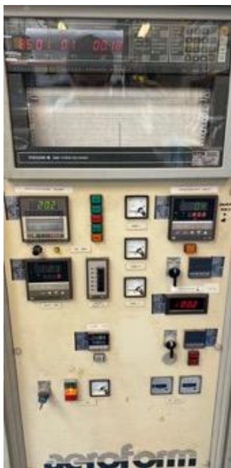
Figure 33: autoclave control panel.
