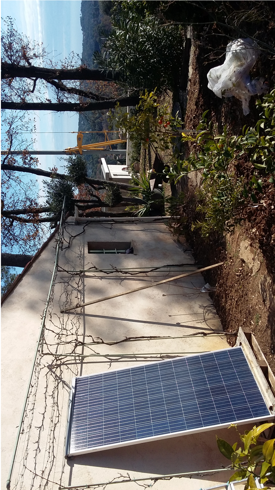
Fig. .58: 300W solar panel in position used for testing
