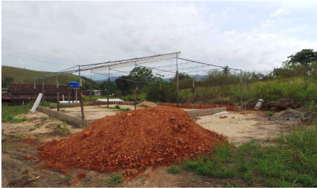
Plate 7.15. Young local Farmer 52 starts construction of a small seedling nursery in November 2017, Tanguá. (Source: Author, 2017)
