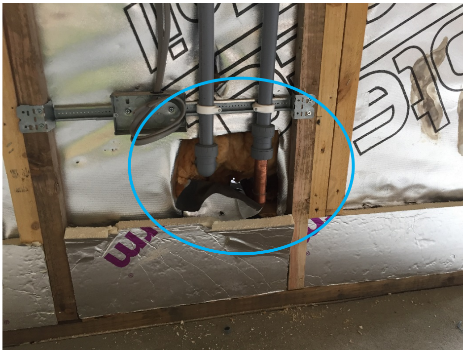
Figure 4-40 Discontinuity of insulation layer and ruptures of vapour control membrane in Case study 1 (Source: Taken by this thesis' author)
