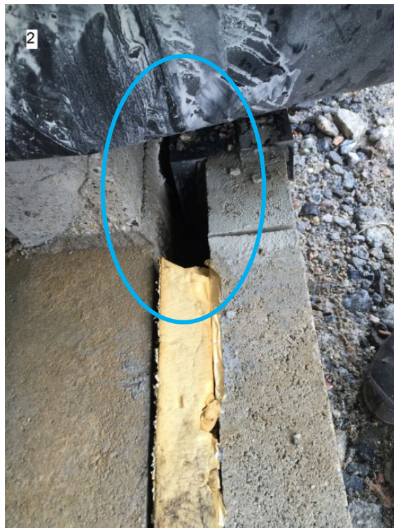
Figure 3-21 Picture 2: Insulation layer between slab perimeter and external wall partially missing
