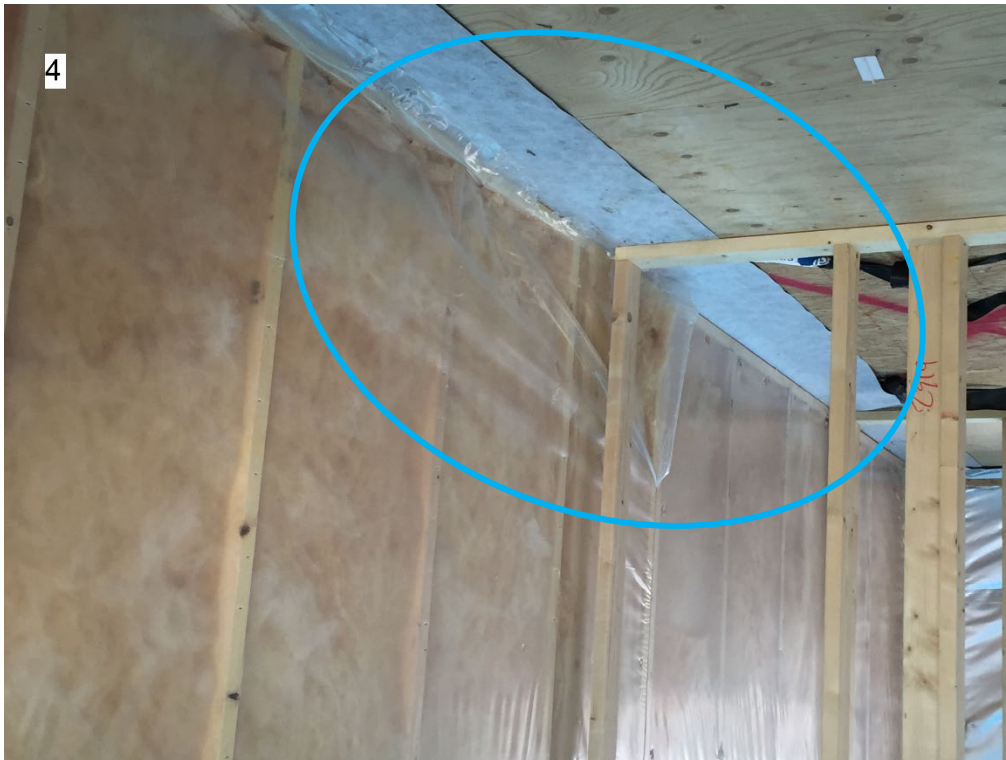
Figure 3-23 Picture4: Vapour barrier of party wall poorly installed
