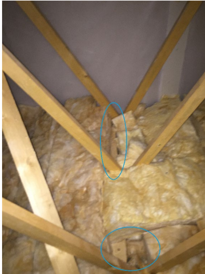
Figure 4-17 Remaining insulation discontinuity defect spotted at pre-handover stage of Case study 2 (Source: Taken by this thesis' author)
