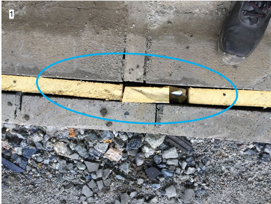
Figure 3-20 Picture 1: Ill fitted insulation boards between slab perimeter and external wall
