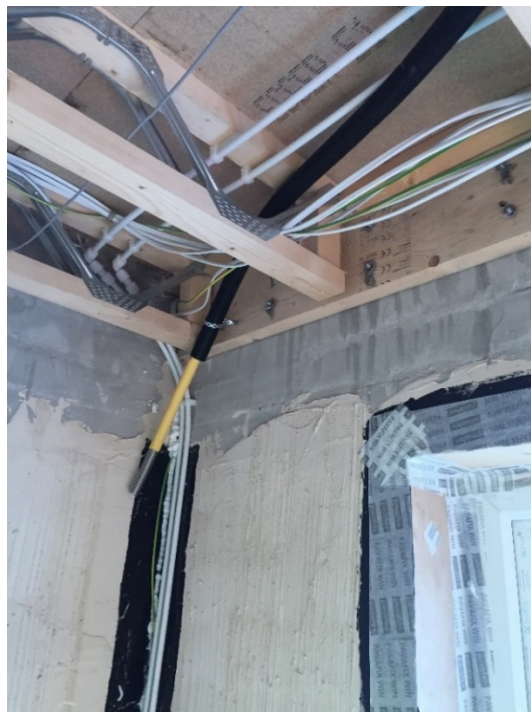
Figure 4-34 Defect potentially affecting air tightness undetected (Source: Taken by this thesis' author)
