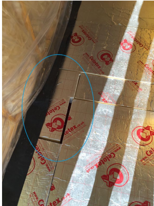
Figure 4-11 Discontinuity of insulation layer identified in Case study 3 (Source: Taken by this thesis' author)
