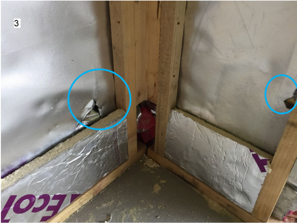
Figure 3-22 Picture 3: Ruptures in vapour control layer
