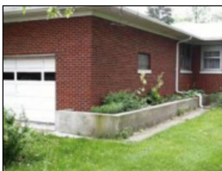
Figure 21: Additional external wall for flood protection (California Department of Water Resources, n.d.)
