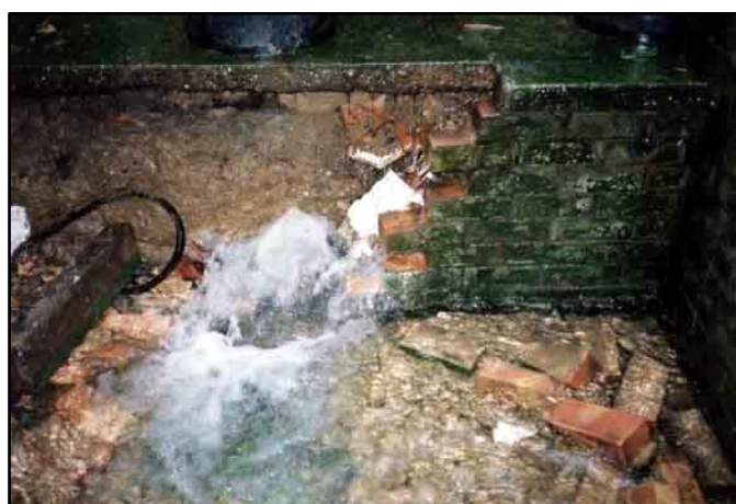
Figure 1: Brickwork wall broken from behind by flood water in Malton, U.K. (Kelman, 2000)
