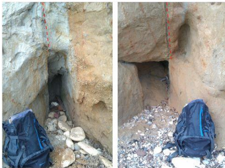
Figure 4.3 Gullies forming where there is a thicker clay horizon, located left of the red dotted line.
