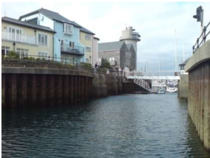
Plate 2. View from the inner marina at Port Pendennis towards the lock gate and outer marina, restricting the water flow.
