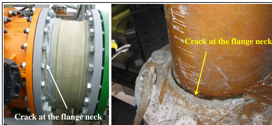
Fig. 4.5: Common failure on the GFRP flanges [33]
