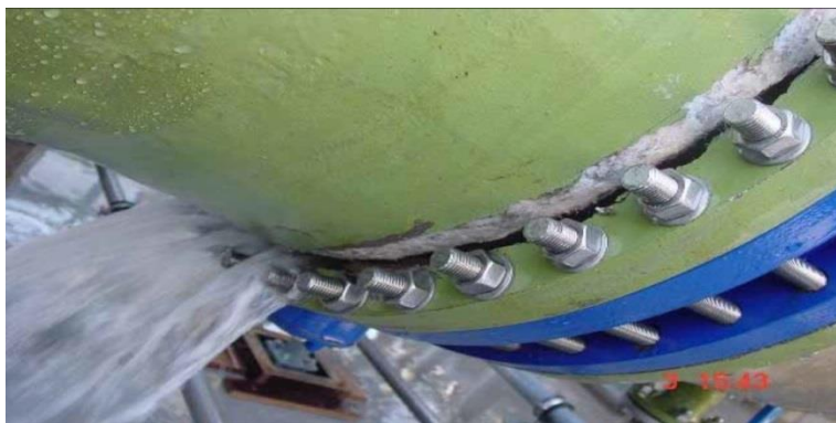
Fig. 2.6: Flange failure at the flange neck [33]
