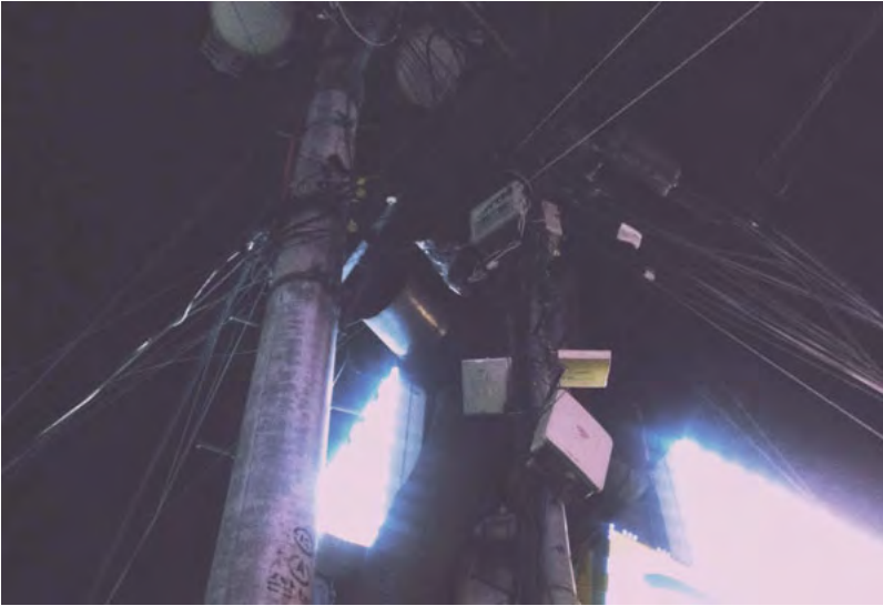
Figure 2. Messy electricity wires and WiFi routers in Seoul.
