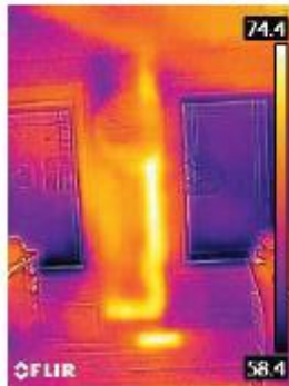
Warm Drain Pipe in Wall
