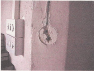
Figure 40 Warmwell, overskim plaster stopped at the edges of a relatively modern light fitting.
