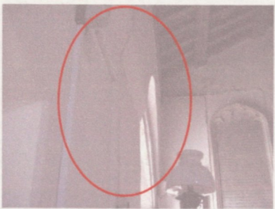
Figure 48 West Knighton. Upper areas of the south wall of the nave showing greatly thickened areas of plaster.
