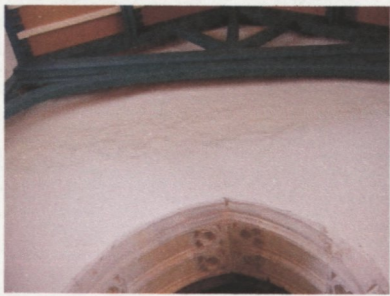
Figure 47 Upwey. Sudden change in the waviness of the plaster above the tower arch.
