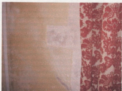
Figure 53 Puncknowle. Damp stains on flat plaster that were initially interpreted as waviness.
