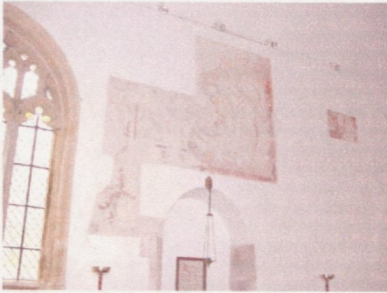
Figure 44 Winterbourne Steepleton. Neat but probably incomplete exposure of wall paintings.
