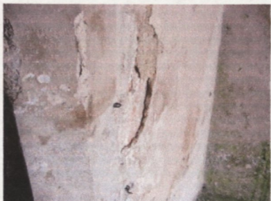
Figure 42 Litton Cheyney. Layers of plaster separated by salt damage. Are they significantly different in date?
