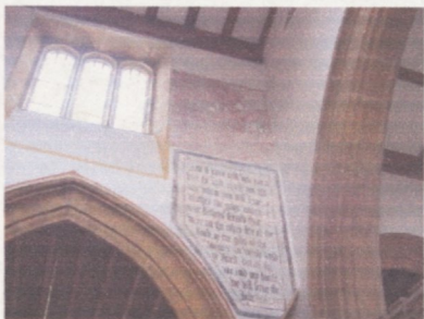
Figure 43 : Cerne Abbas. The upper area of exposed medieval painted plaster appears too neat an regular to represent the full extent of the survival.
