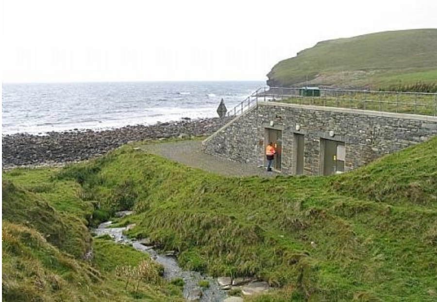
Figure 6: EMEC substation external view.
