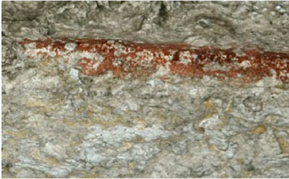
Figure 56: Close up of remaining paint
